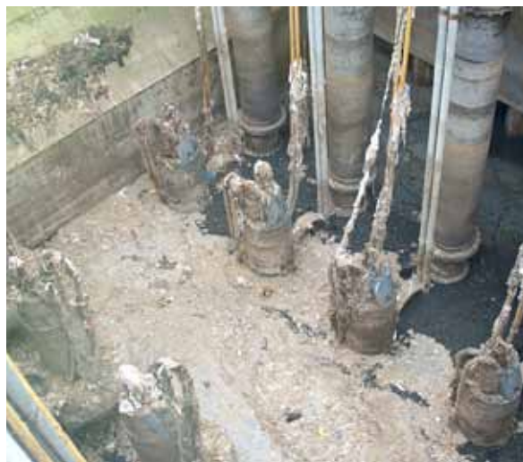
Pump station with accumulation of floating debris.
