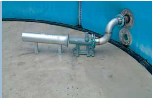
Inside the tank: The nozzle and ejector pipe are located to generate a bulk flow loop, which leads to re-suspension and homogenization of the mixed sludge.
